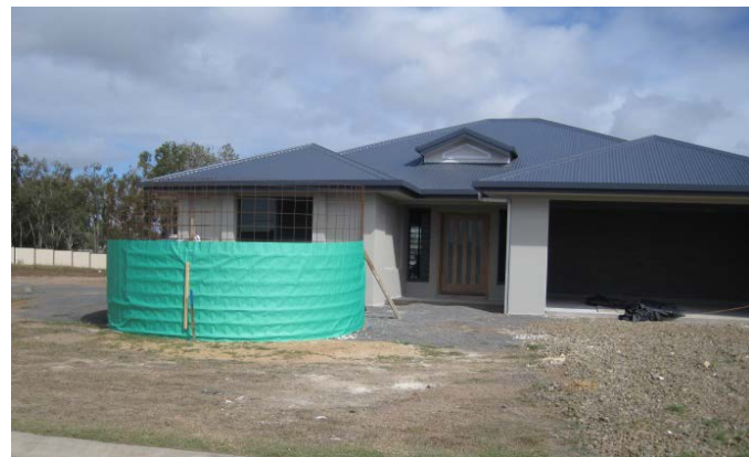
Figure 1 - A waste enclosure with a shade cloth surround to stop all waste being blown off site
