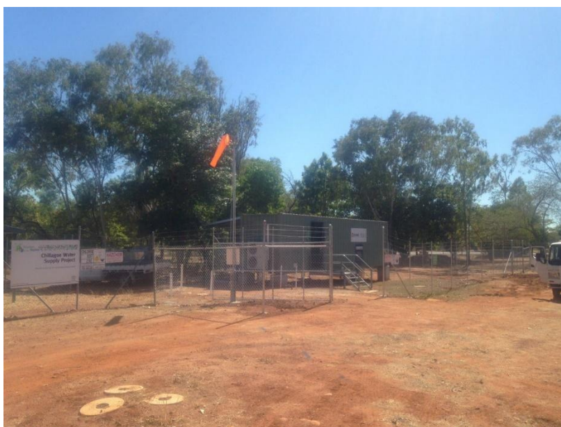
FIGURE 3: CHILLAGOE WATER TREATMENT PLANT
