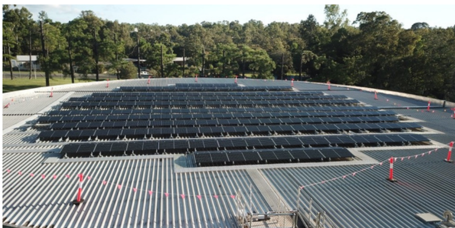
Solar installation Mareeba water treatment plant
