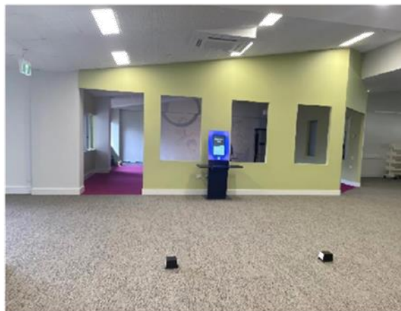
Power and data installed for new PC area in foreground, self-check kiosk for borrowing and quiet reading area in background
