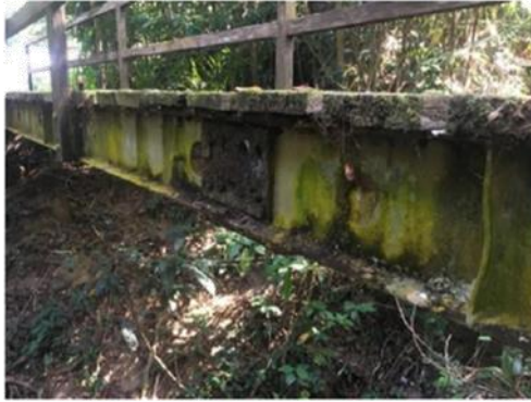
Old Barang St Pedestrian Bridge - corrosion
