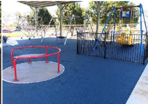
Completed section with damaged soft fall
