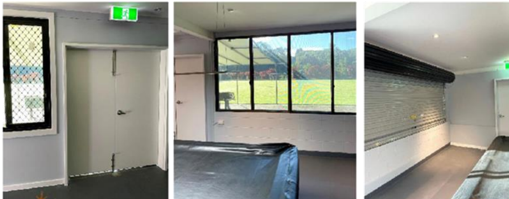
Ground floor: Refurbishments undertaken including waterproofing, new fire doors and roller doors
