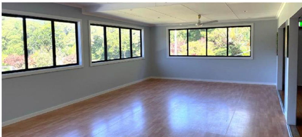
First floor: Completion of refurbishment, including installation of new windows and painting
