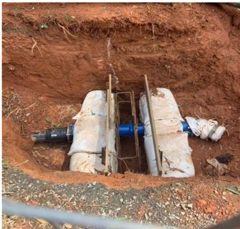
Cut in and laying new discharge and suction lines to the new booster pump station
