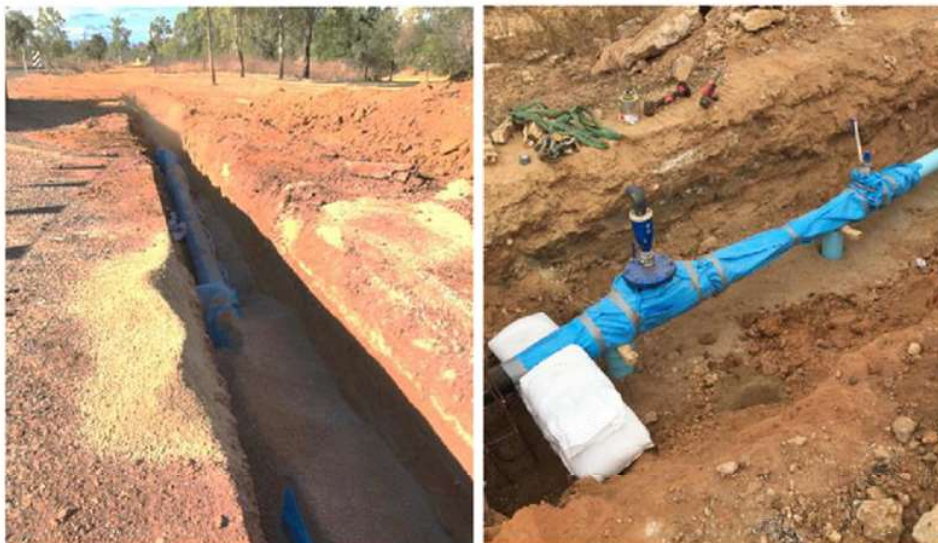
Newly road crossing pipeline in DICL construction and pipeline air release valve
