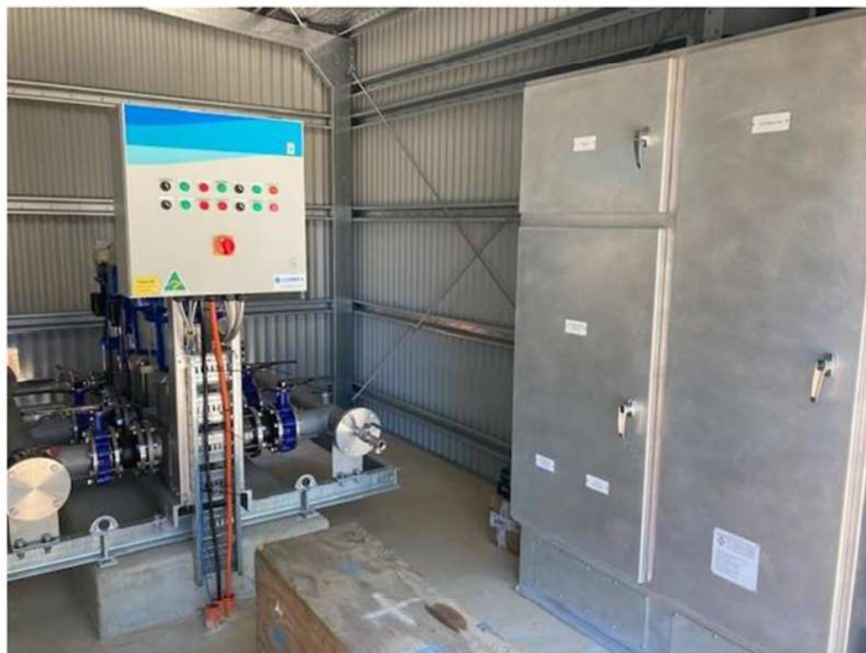
Newly installed booster pump set and electrical switchboard which incorporates SCADA & Telemetry
