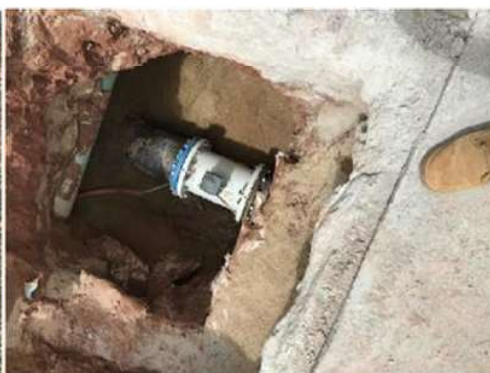
Newly installed flow meter
