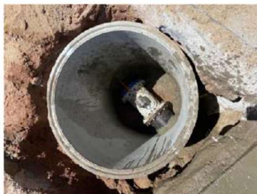
Newly installed access chamber with class D trafficable cover to be fitted
