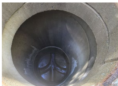
Before Water and root ingress into manhole
