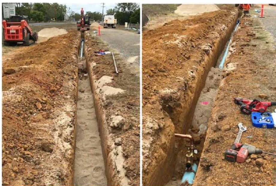
Laying and installation of the new 150mm diameter PVC Supermain water main
