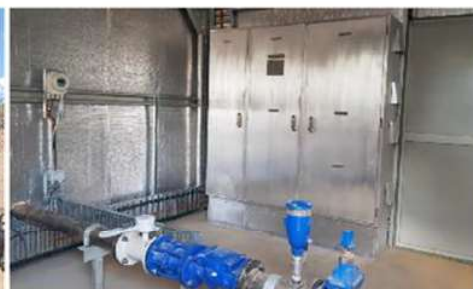
Newly installed standby generator for the Bore & Telemetry
