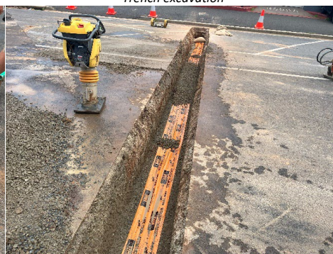
Conduit protective cover
