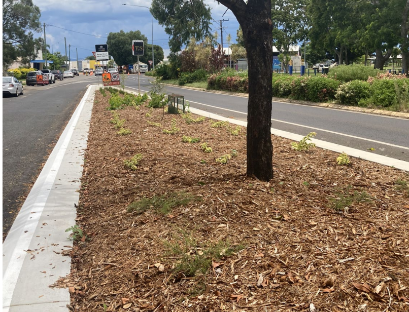
Location 8 Byrnes Street Median Island on the eastern side of the road between Railway Avenue (northern end) and Granite Creek. Construction complete.
