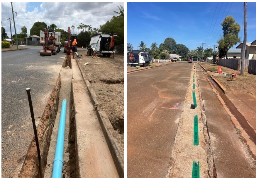
Keeble Street and Adams Street installation of the new 150mm diameter PVC Supermain water main
