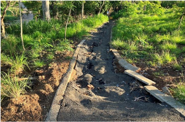
Granite Creek Asphalt Path – 08/01/2024
