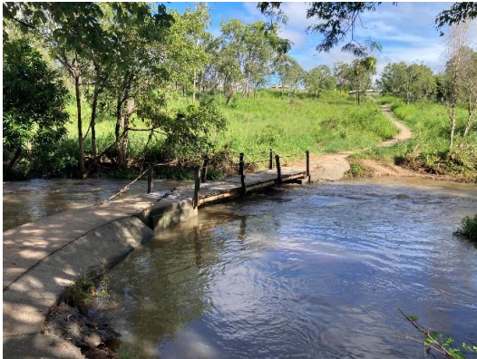
Pedestrian bridge before repair
