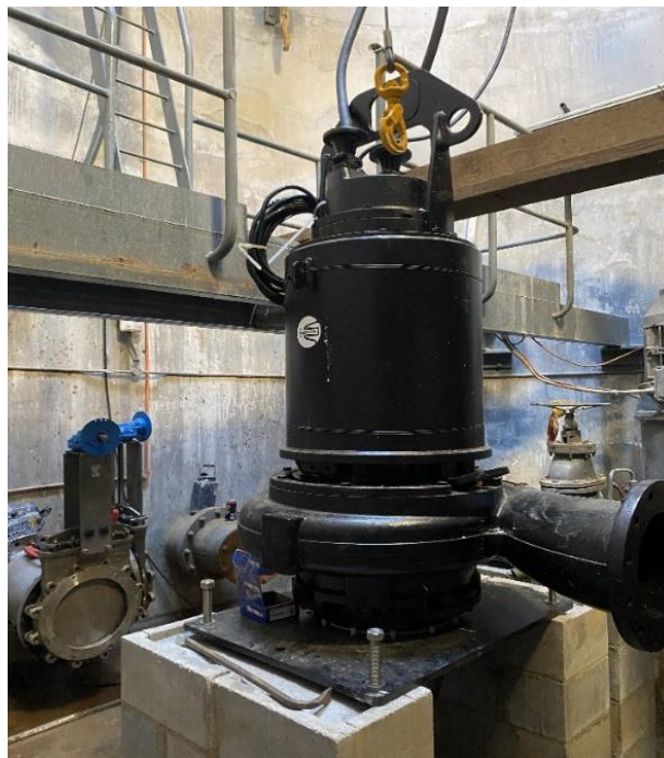
Stripping out the old pumps and pipe work to make way for new infrastructure.
