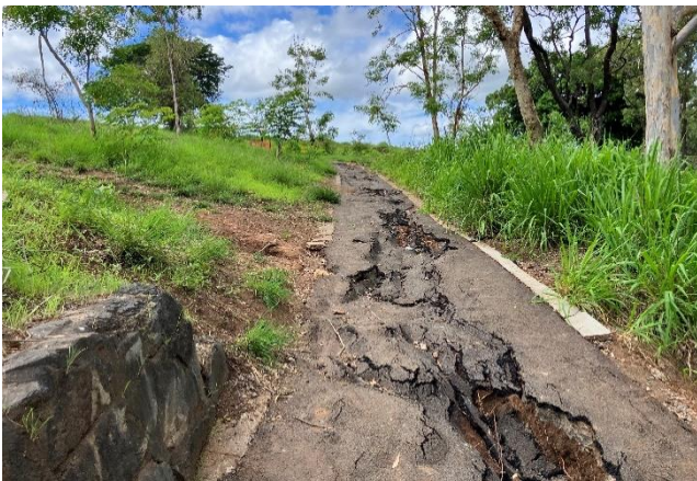
Granite Creek Asphalt Path – 08/01/2024
