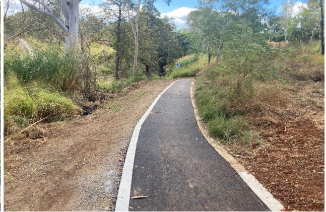
Granite Creek Asphalt path – 26/06/2024
