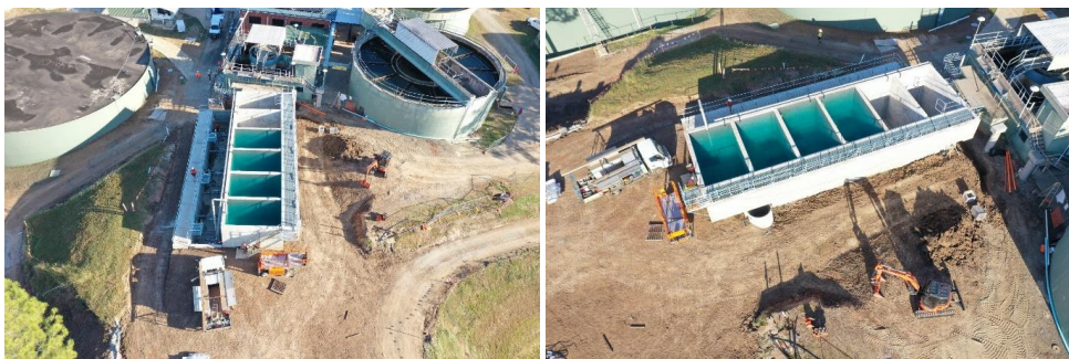
Concrete construction of new filter cell modules and installation of new pipe work and earth works to back fill around the filtration modules.
