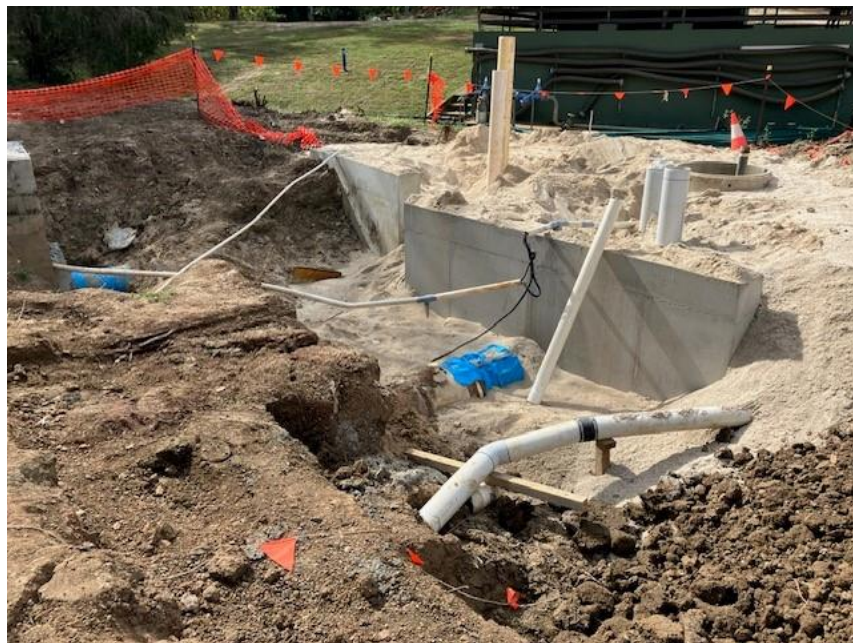
Site construction works and concrete plinth for booster pumps to be mounted onto.
