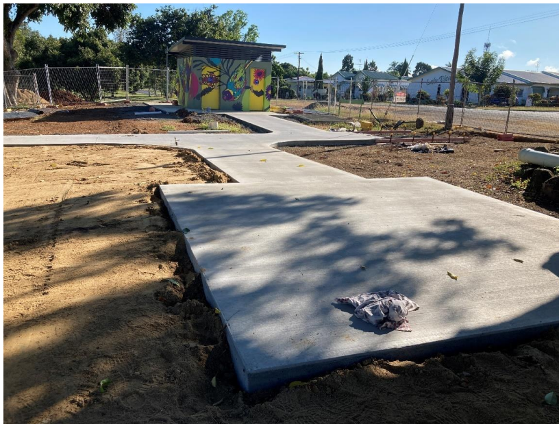
Bicentennial Lakes Mason Street New Public Toilet, footpaths and picnic shelter pad construction
