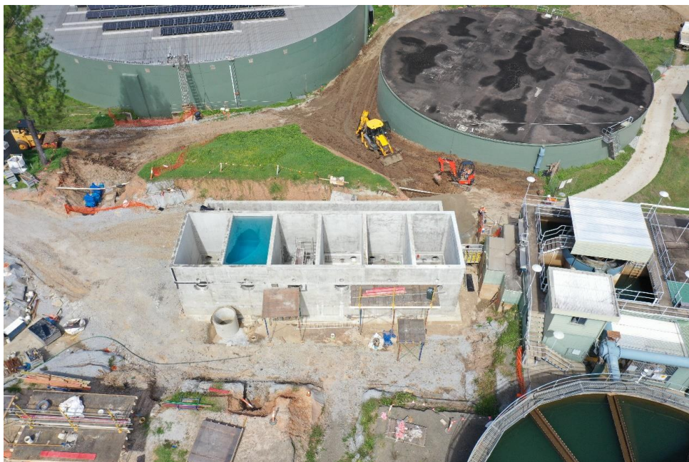
Concrete construction of new filter cell modules and installation of new pipe work
