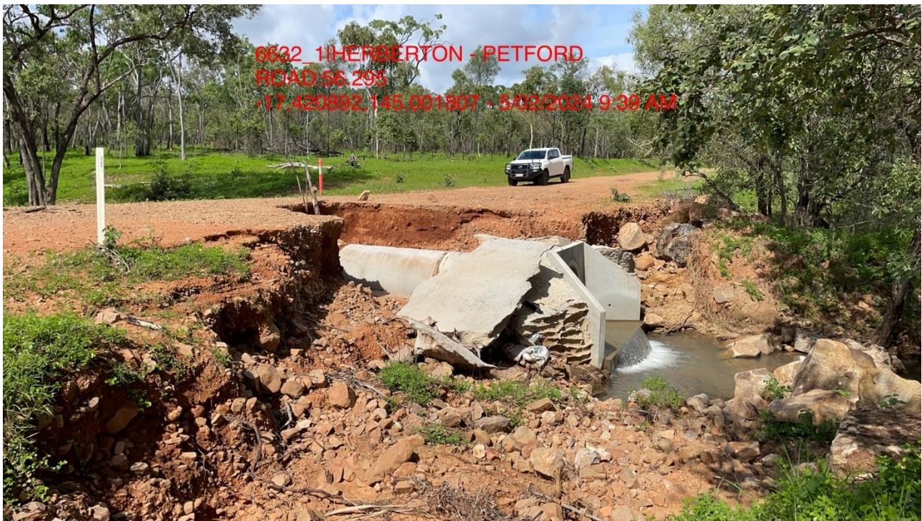
Culvert washout on Herberton-Petford Road
