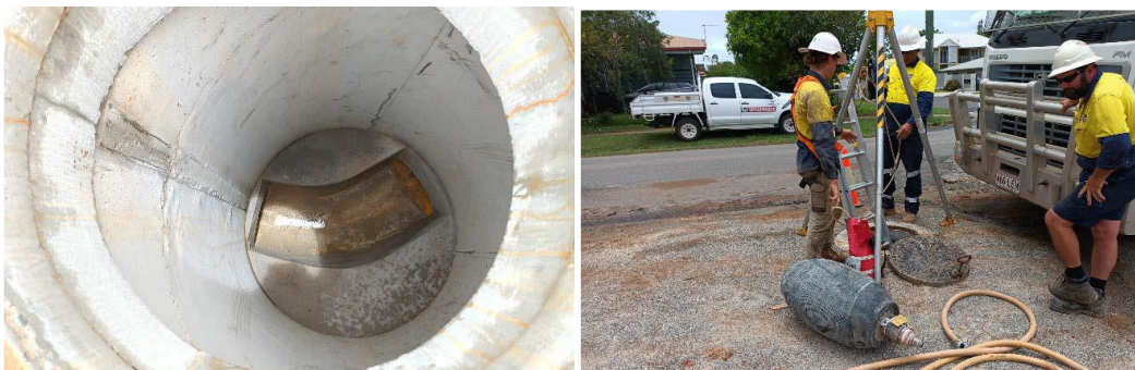
Completed manhole benching in manhole 1/11 and confined space entry works for air testing of pipeline sections
