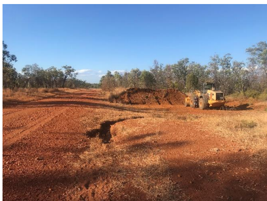
Road reserve stockpile
