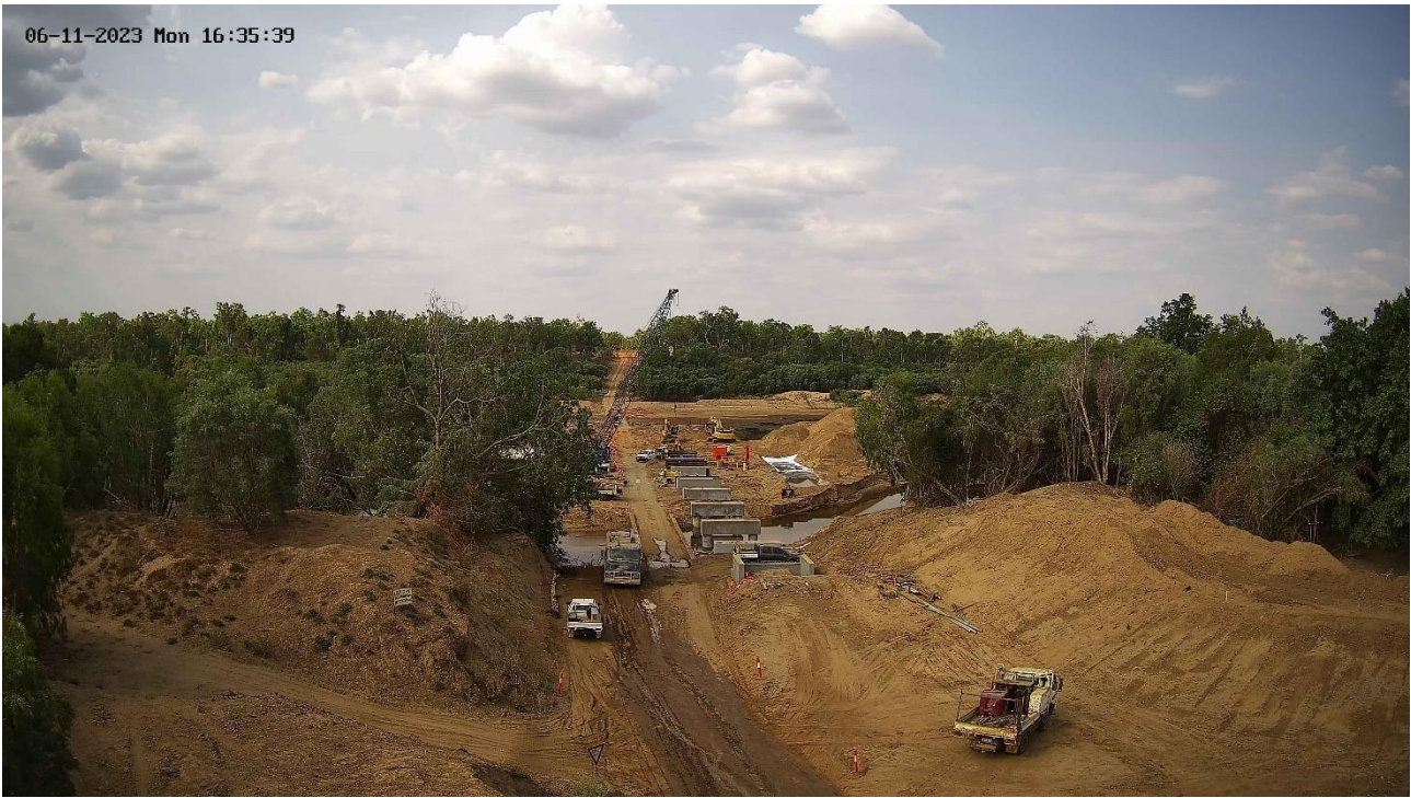
Gamboola Crossing over Mitchell River, Strathleven Road – construction of bridge piers and headstocks in progress
