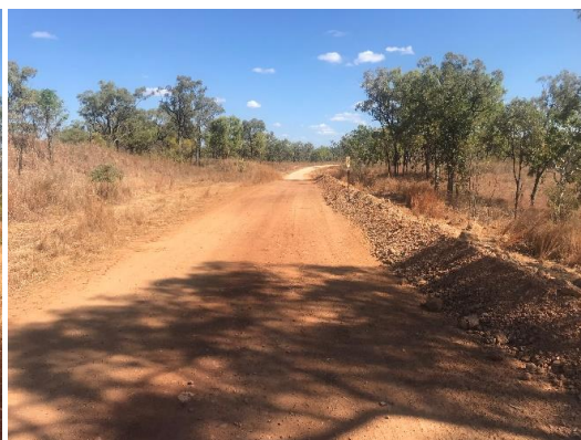
Rilled re-sheeting material
