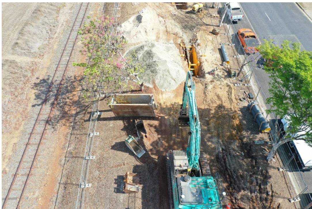
Sewer installation on the verge between Queensland Rail line and Railway Avenue.
