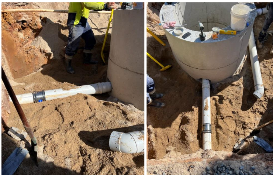
Existing DN150 sewer installation through new manhole, existing sewer to be cut inside manhole once new sewer line is commissioned
