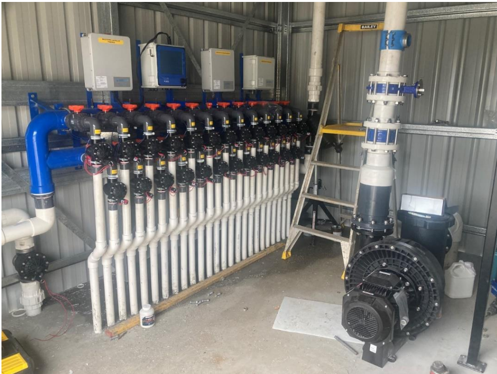
Splash Park Filtration Shed
