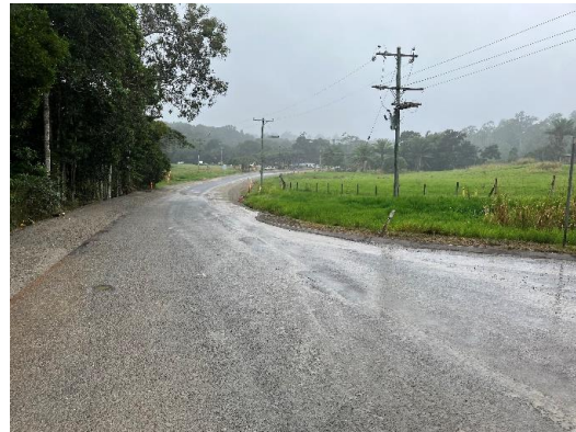
Works yet to be sealed
