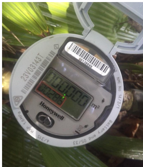
A new fully integrated smart meter that was recently installed in Kuranda.
