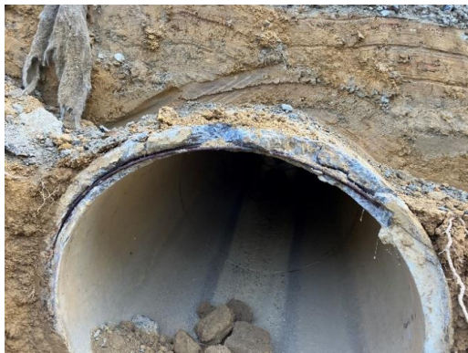
Failing 1050Ø pipework (Ch 9479)
