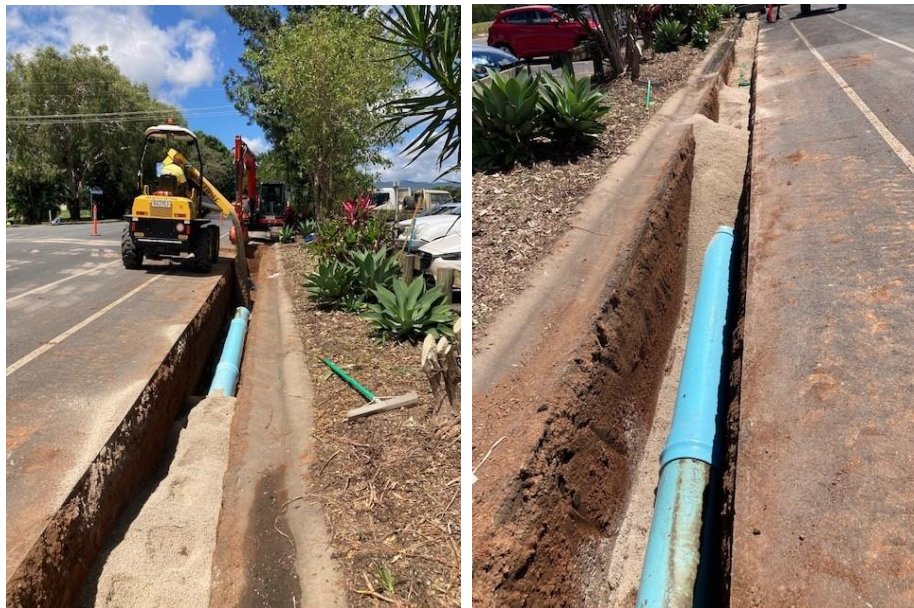
Anzac Avenue installation of the new 300mm diameter PVC Supermain water main
