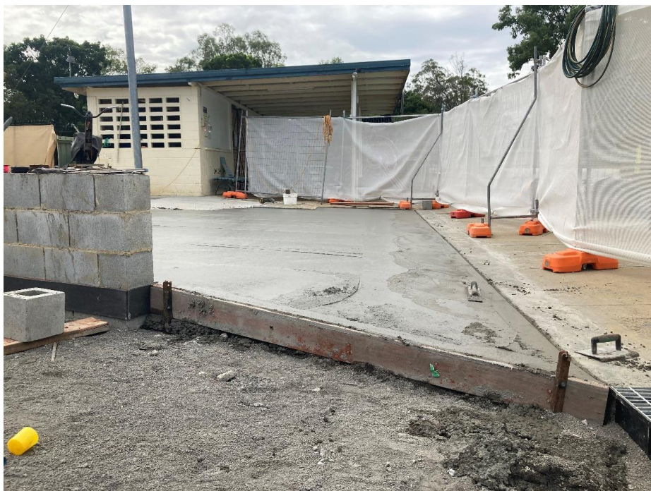
Existing pavers replaced with new concrete between old clubhouse, 50m pool and new Splash Park
