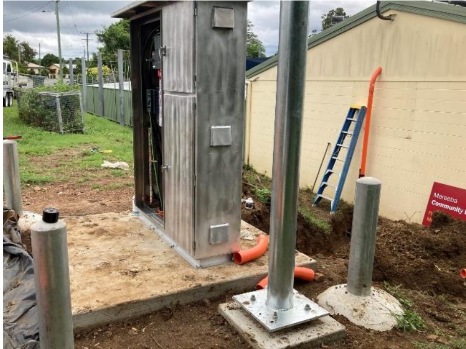
Ergon Energy Transformer Upgrade
