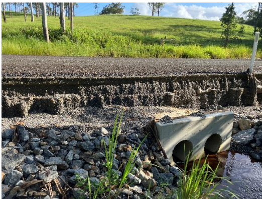
Culvert outlet damage
