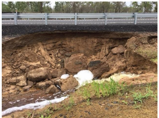
Erosion on Mareeba – Dimbulah Road
