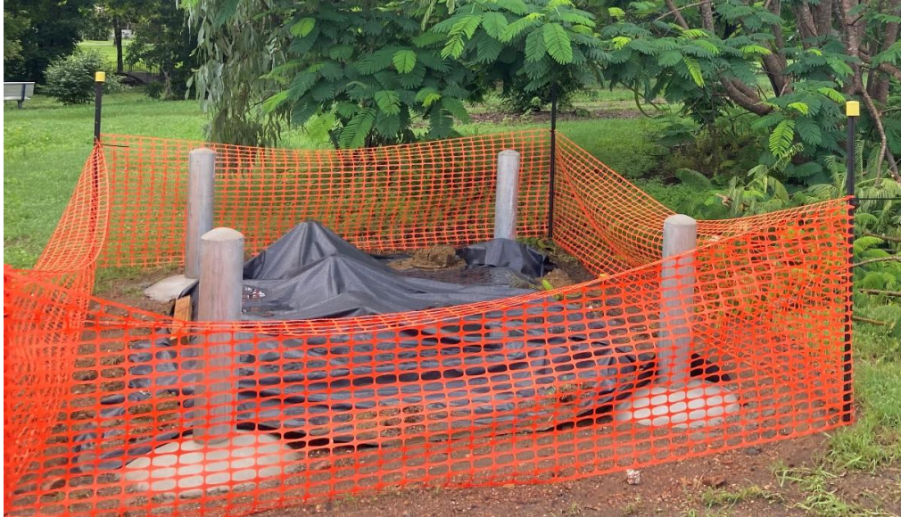
Mareeba Aquatic Centre Ergon Energy Transformer Upgrade
