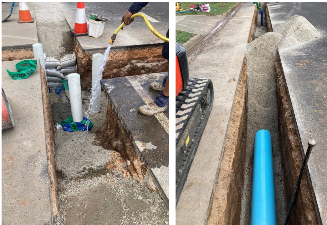
Anzac Avenue installation of the new 300mm diameter PVC Supermain water main
