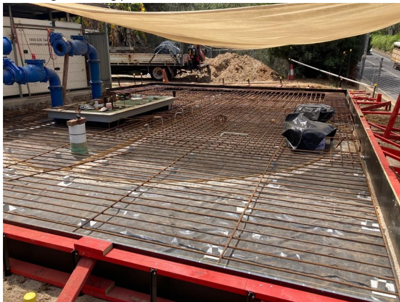
New pump station concrete top being set up ready for concrete pour
