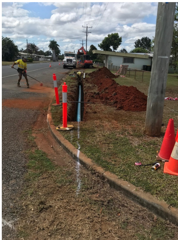
Installation of the new 150mm diameter PVC Supermain water main along Chewko Road
