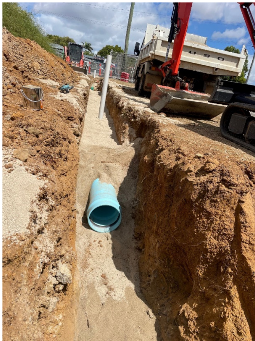
Herberton Street installation of the new 300mm diameter PVC Supermain water main
