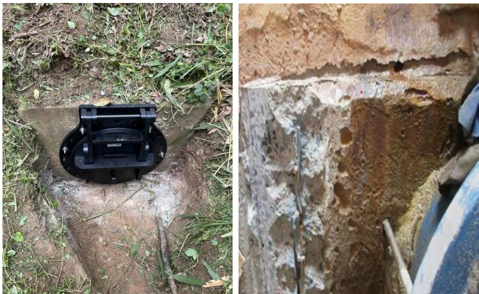
Installation of a frog flap to the overflow line to the licenced discharge point and internal wall scalping
