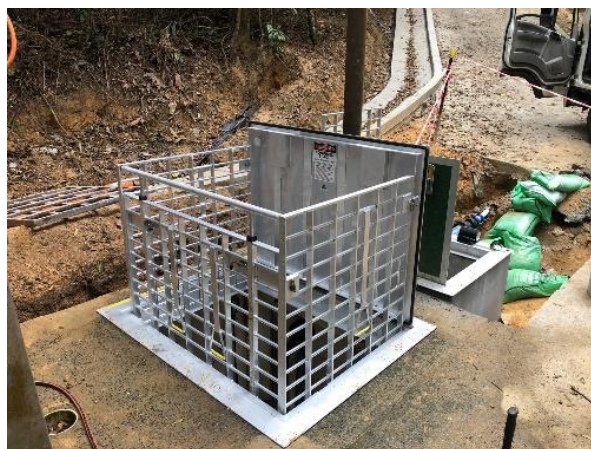
Thooree Street SPS valve pit and wet well lids installed, sealed and grouted
