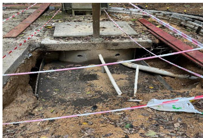
Excavation and core hole penetration into the pump station to allow for new discharge pipework
