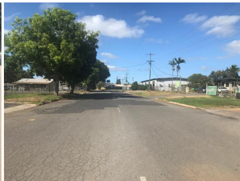
Aged and cracked asphalt
