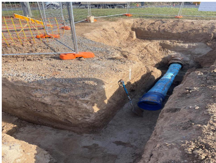
Installations of the new 300mm diameter Ductile Iron DICL water main at Vaughan Street
