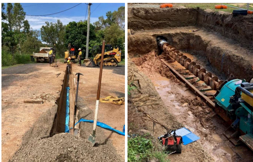
Installations of the new 100mm diameter PVC Supermain water main Starcke Street and under boring from the cemetery entrance under Vaughan Street
