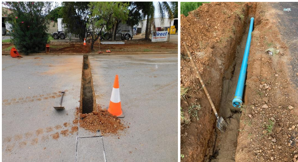
Road crossing and road verge installations of the new 150mm diameter PVC Supermain water main
