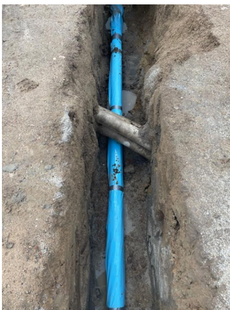
Installations of the new 100mm diameter PVC Supermain water main Starcke Street
