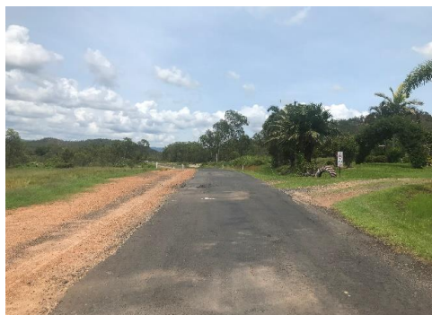
Pavement failure at Ch 7960
