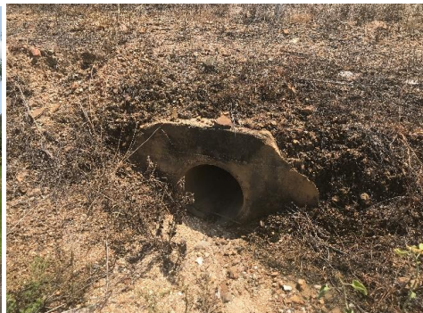
Narrow culvert and failing headwall Ch 8600
