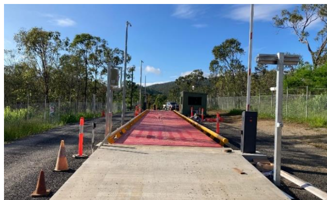
Newly installed Weighbridge
