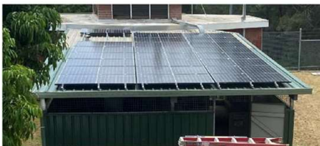
Granite Creek Pump Station
