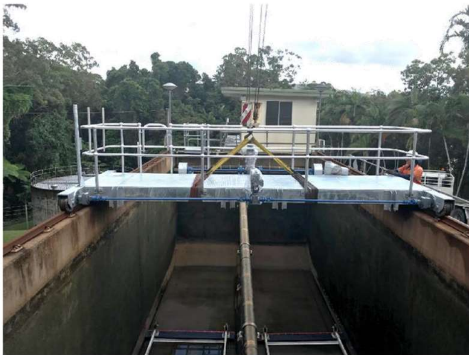
Clarifier trolley assembly
