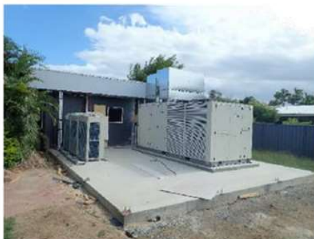
Mechanical Plant installed
