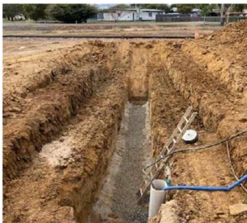
Excavation works to install the section of sewer main under the rail line
