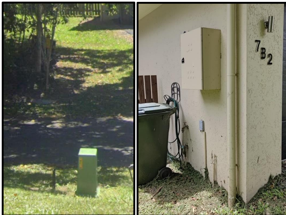
Figure 8: Metered reticulated electrical provisions to existing Dwellings (STP).
