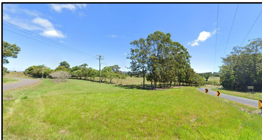
Figure 6: Reticulated electrical provisions, Barnwell / Oak Forest Rd. (Google Maps).
