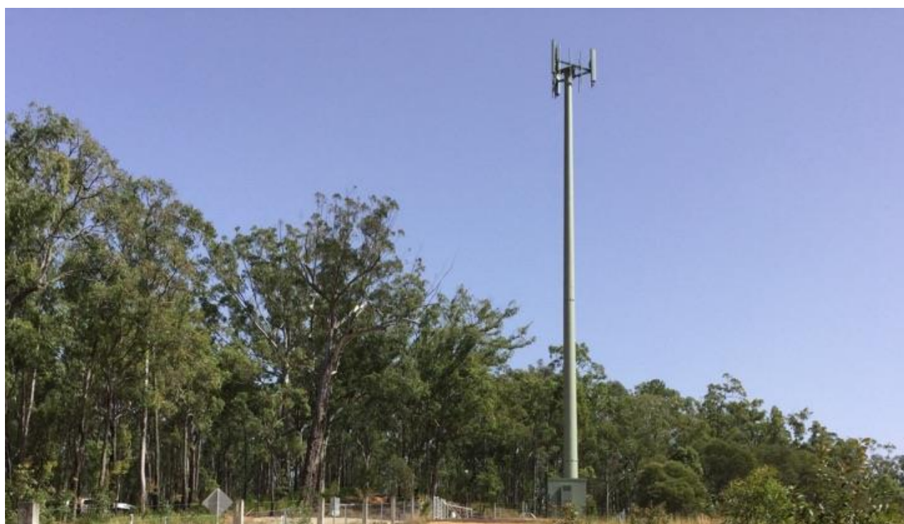
Figure 9: Image of example 40m monopole with headframe and antennas all colour-treated mist-green. Note that image does not include solid coloured fencing surrounding compound (Source: Ventia, 2020)
