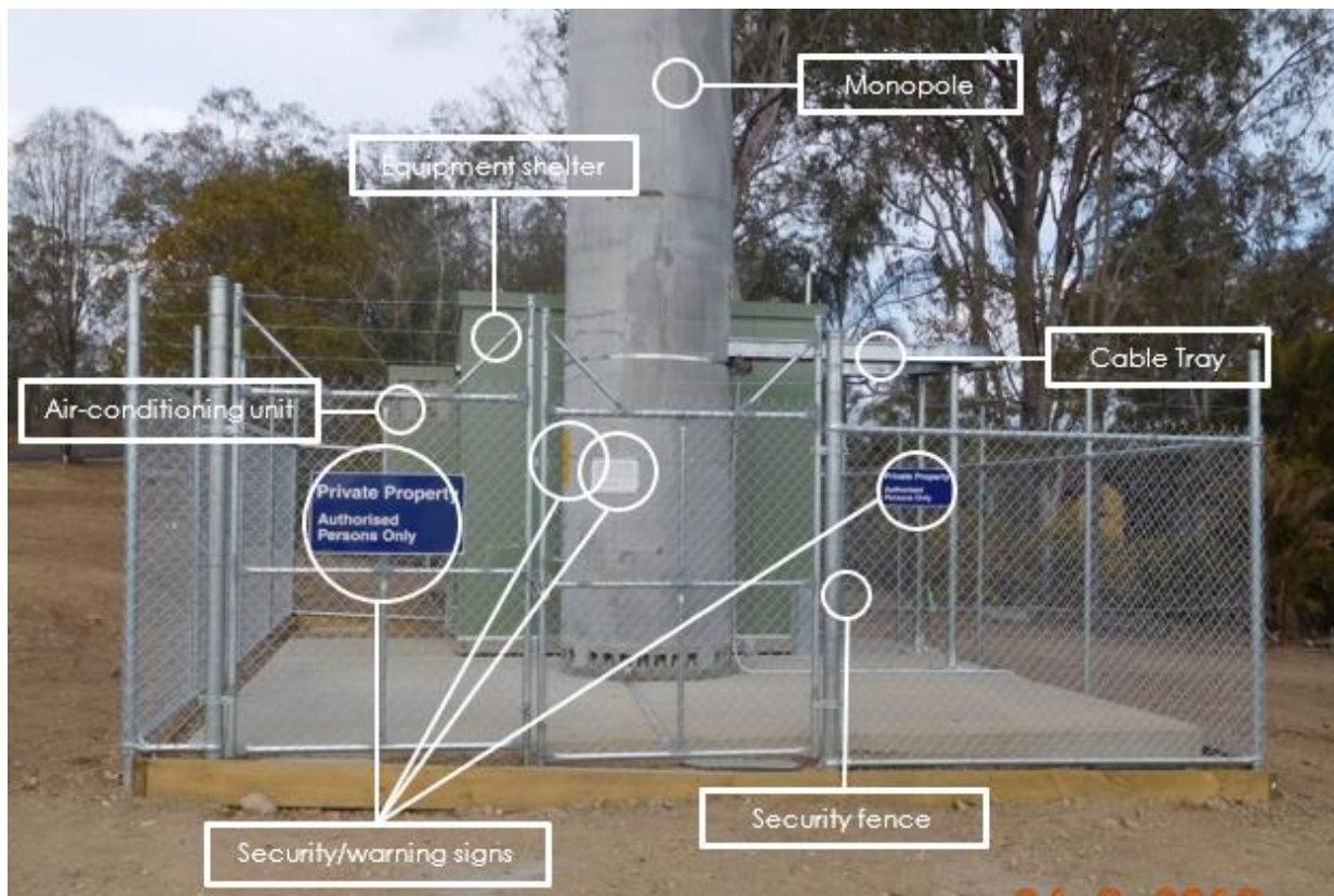
Figure 8: Image of example compound with security fence, equipment shelter cable tray and concrete pole (no-colour-treatment and example does not include solid coloured fencing surrounding compound) (Source: Ventia, 2020)
