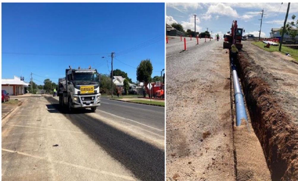
Construction and installation of the new 300mm ductile iron water main and cut-in and valve arrangement at the Rankin Street and Chewko Road intersection.
