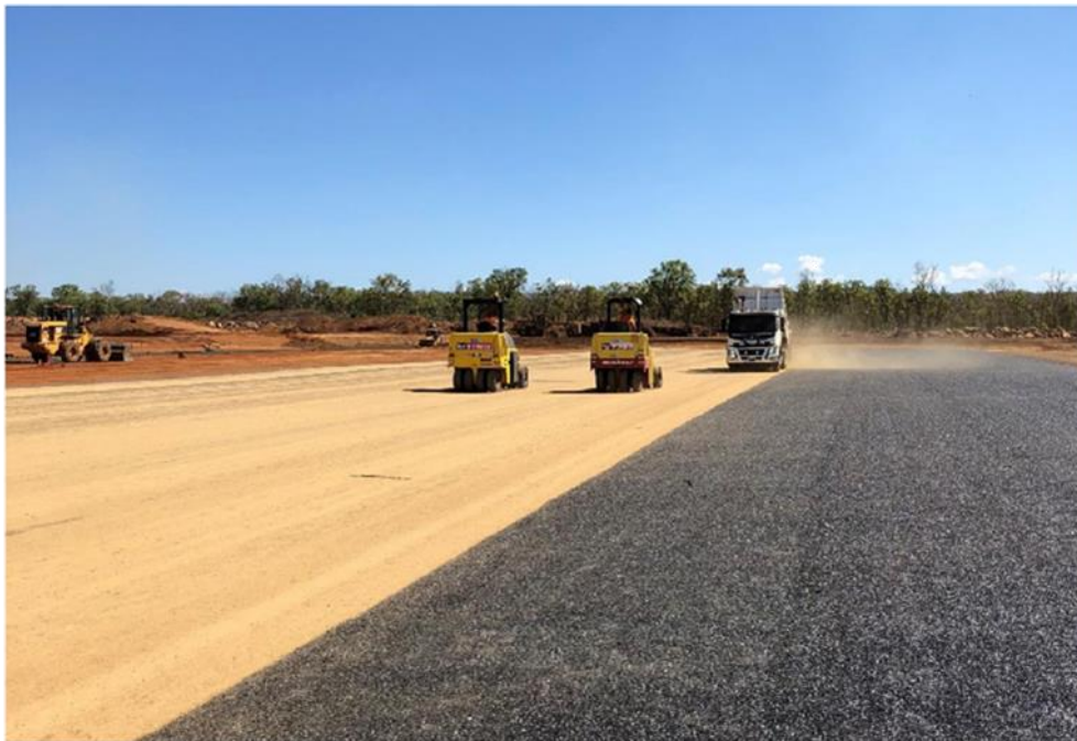
16 November 2018 - spreading and rolling of sand locking coat as part of 3-coat seal to taxilanes and aprons in aviation industrial park
