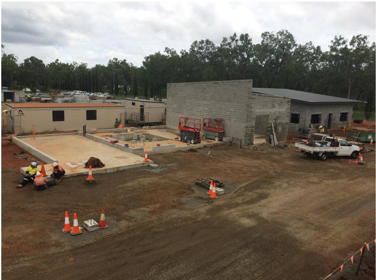
31 January 2017 - Progress on the construction of site buildings with completion of walls to Blower Building
