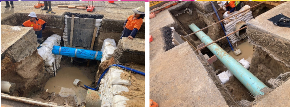
Stormwater Pipe Conflict with Existing Water Main - Ductile Pipe Cut-In & SW Pit Reconfiguration
