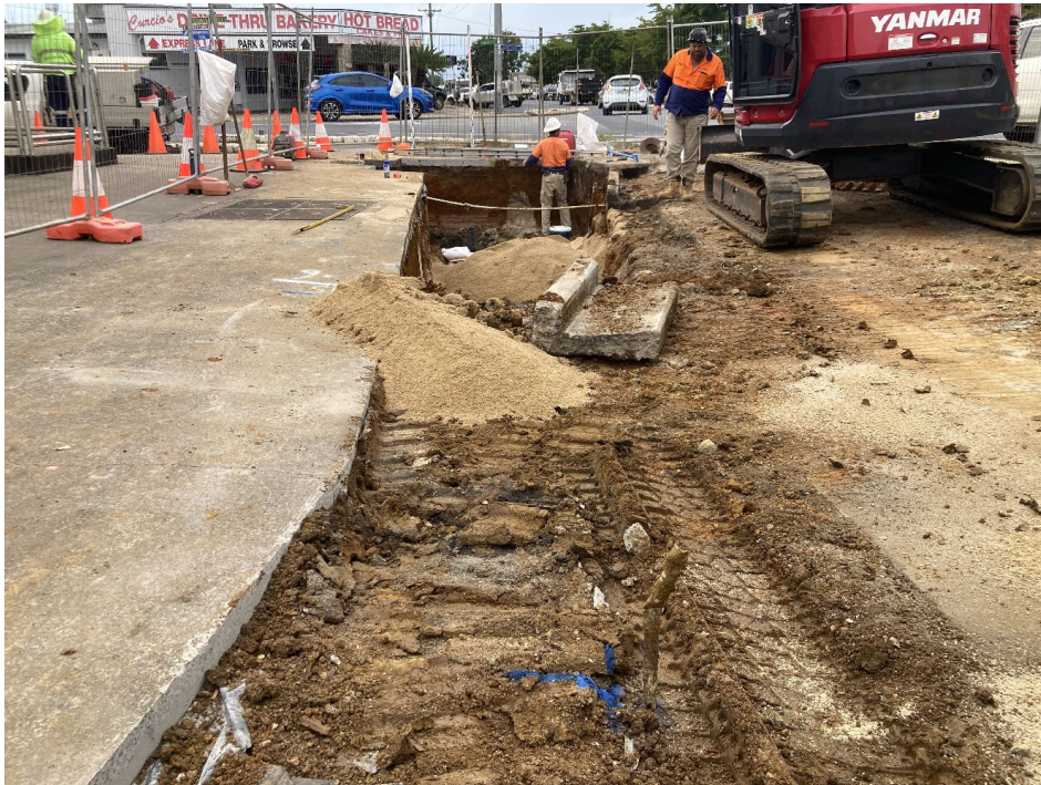
Walsh Street Stormwater Pipe Trenching & Installation Highlighting Ground Conditions and Existing Service Lines
