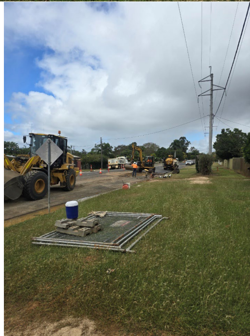
Works on Road crossing and 150mm reticulation Main between Lerra Street and Basalt Street
