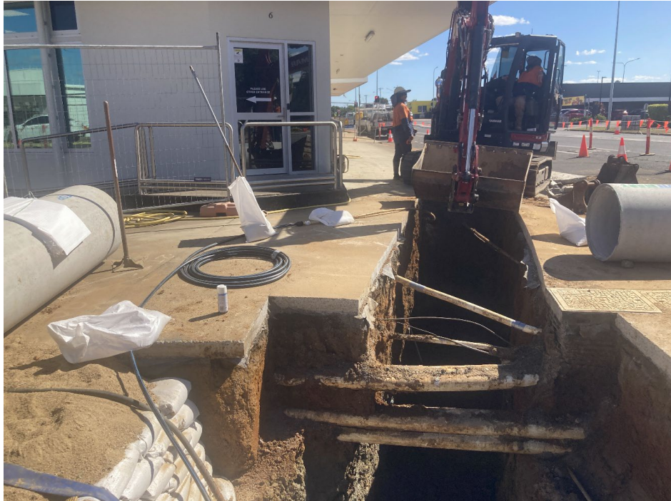
Stormwater installation on corner of Rankin Street and Walsh Street highlighting existing service lines
