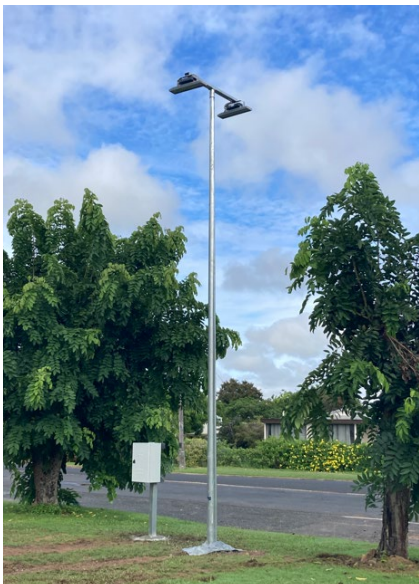
New 8-Metre Lighting Pole
