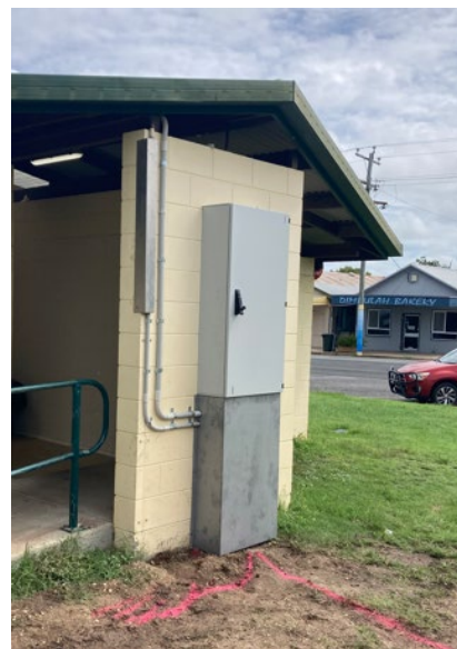
New Main Electrical Distribution board
