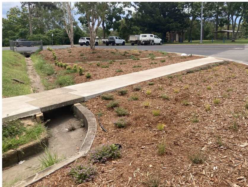
Location 6 (Northern Byrnes St Corner of Railway Avenue and Rotary Park). Construction complete.
