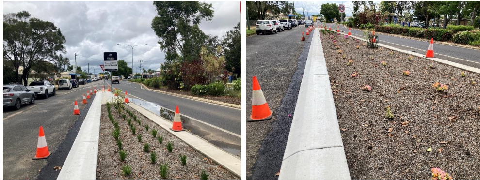
Location 8: Concrete kerbs installed and planting underway on Byrnes Street Median Island on the eastern side of the road between Railway Avenue (northern end) and Granite Creek
