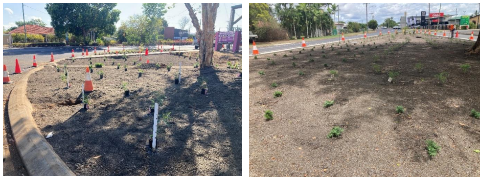
Location 6 (Northern Byrnes St Corner of Railway Avenue and Rotary Par) and Location 2 - BP Median Island: Concrete kerbs installed and planting underway.
