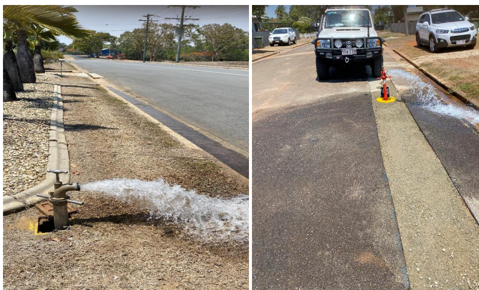
Keeble Street and Adams Street installation of the new 150mm diameter PVC Super-main water main completed
