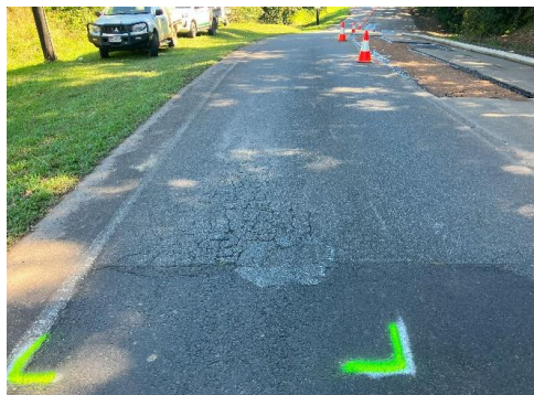
Milling of failed section near Jarawee Road intersection
