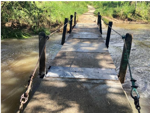
Pedestrian bridge before repair
