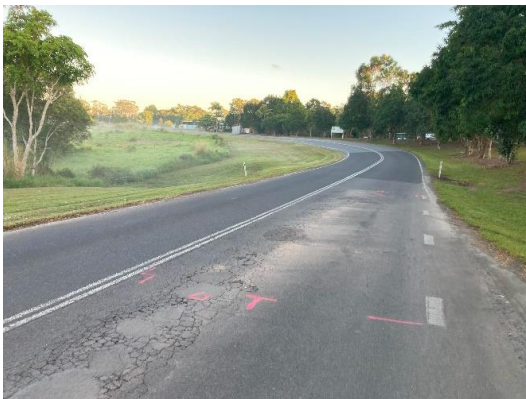
Example of pavement failure on Myola Road
