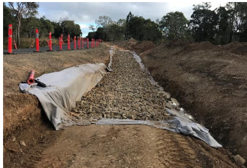
Bidum and rock unsuitable subgrade treatment
