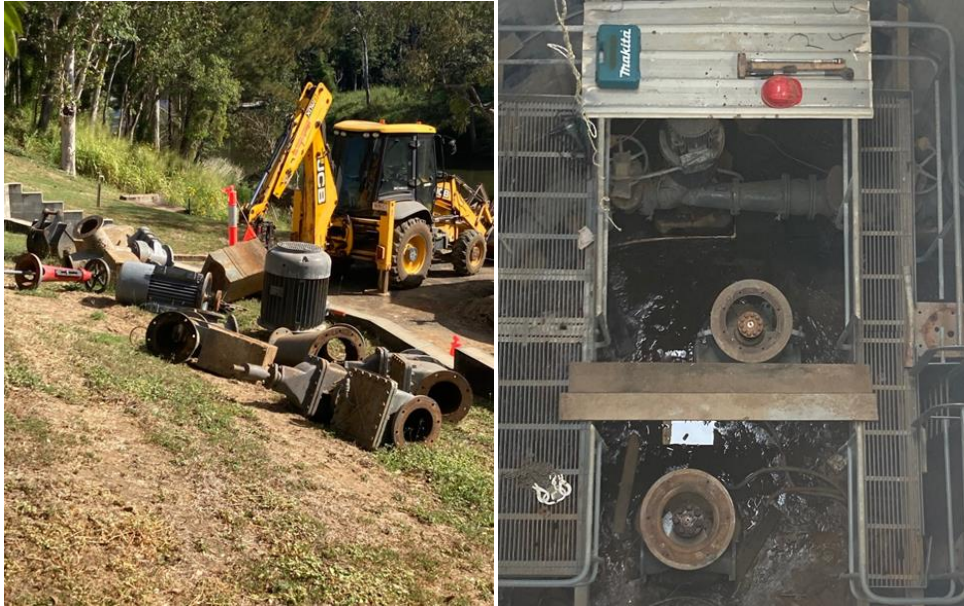
Civil Stripping out the old pumps and pipe work to make way for new infrastructure.
