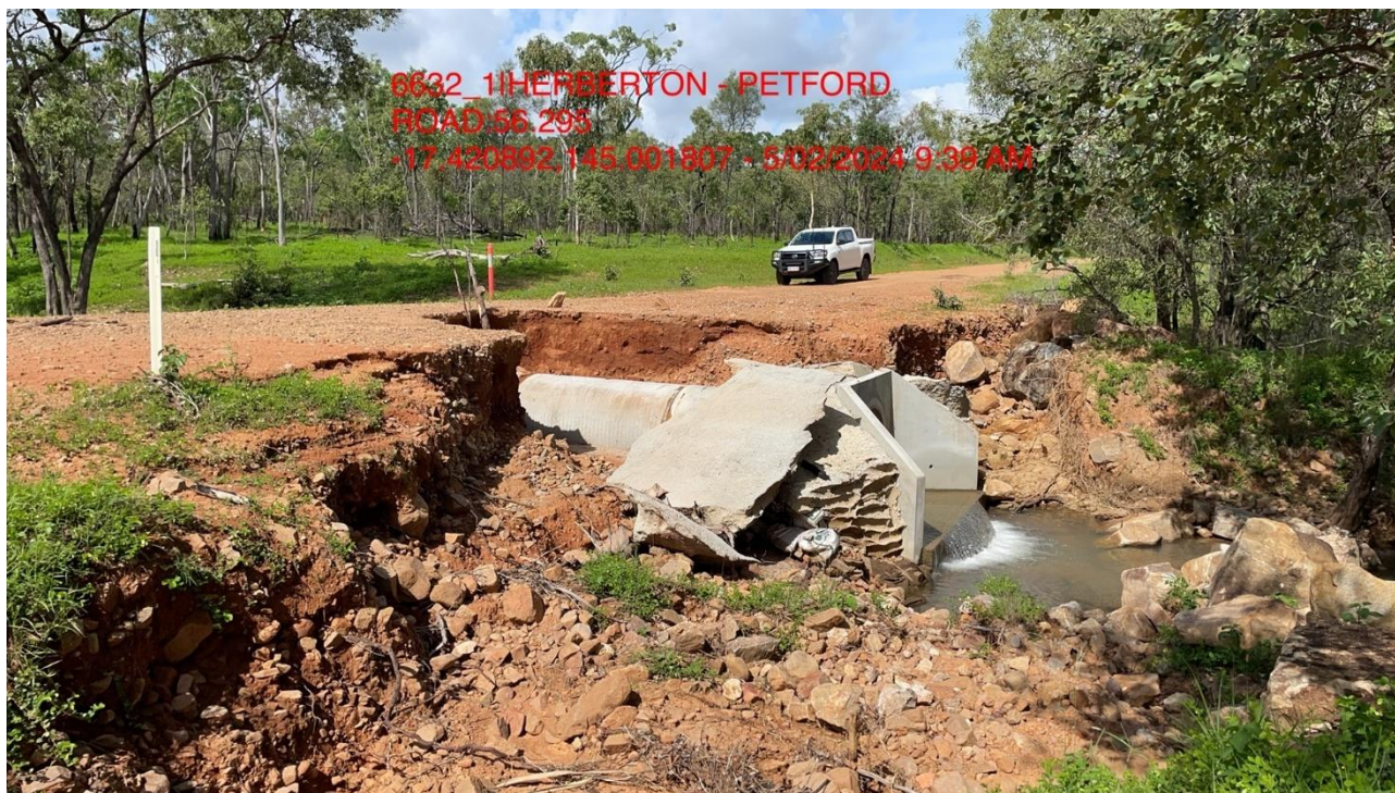
Culvert washout on Herberton-Petford Road
